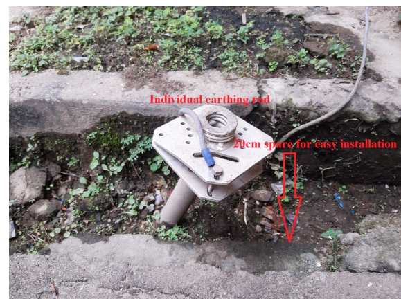
Fig. 3. Individual earthing rod that is wired to the motor frame with 20 cm spare length for easy installation
