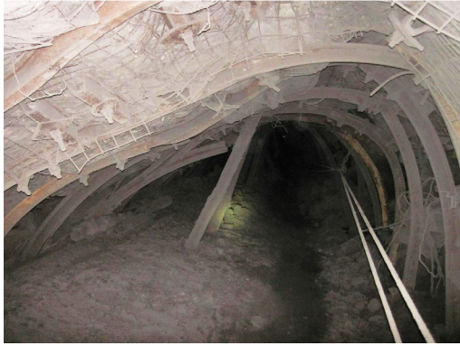
Fig. 1. Development of the mine working contour displacements
