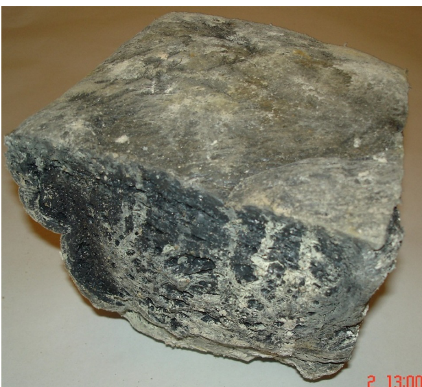
Fig. 2. A sample of concrete with applied polymer compound coat based on the secondary materials after testing under the corrosive environment conditions in camera No. 2 of the sewer in Kharkiv
